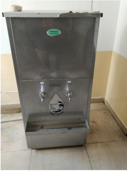
Fig 1. water coolers installed in the buildings
